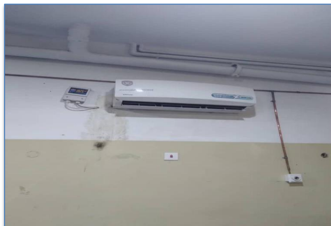
Figure 1: Air conditioner in a service user dormitory
